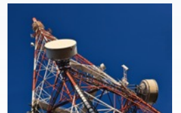
Telecom backup power
